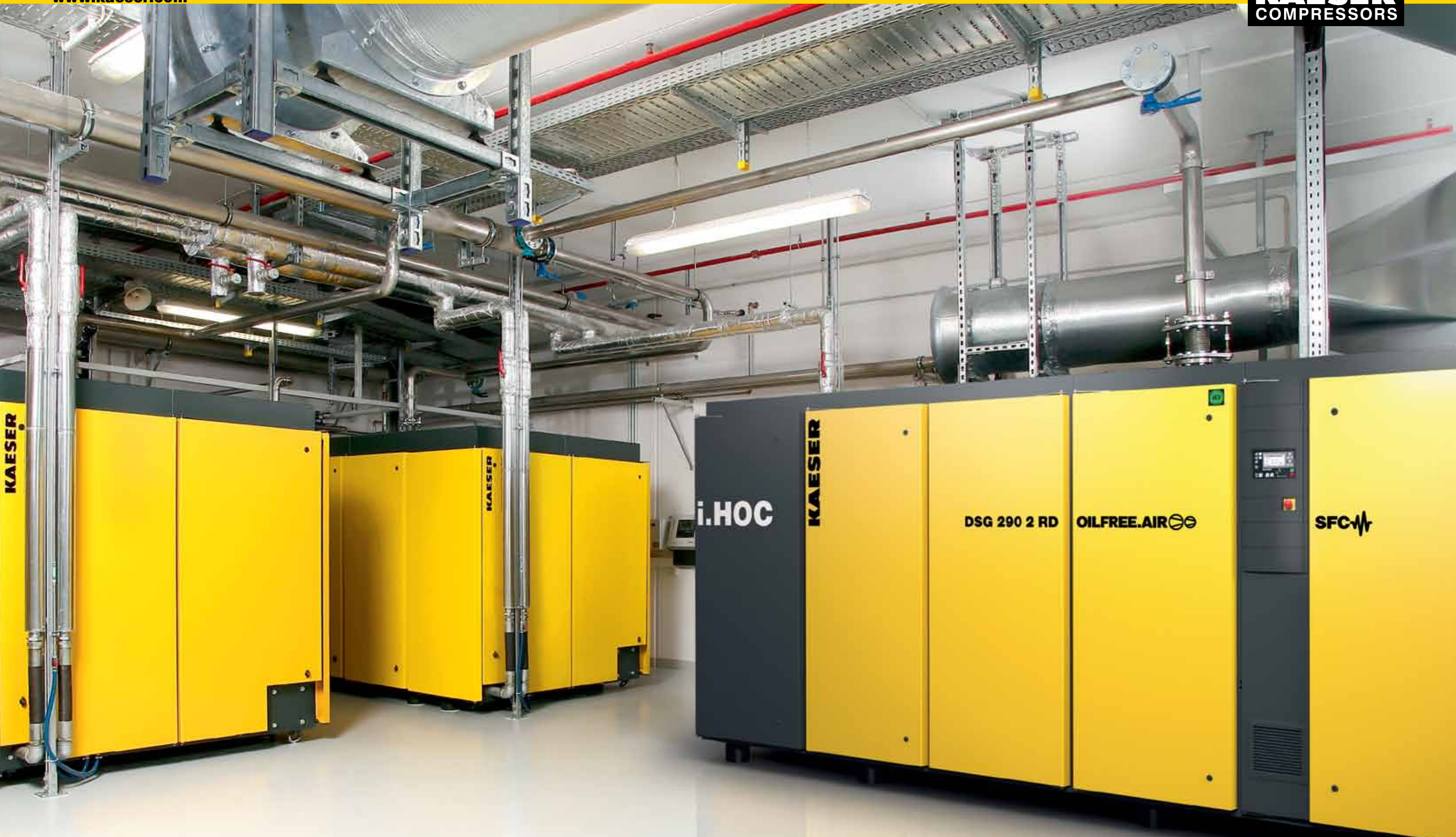
Image: Example of a KAESER station that has been expanded with the installation of a water-cooled DSG 290-2 RD SFC dry-running rotary screw compressor.
